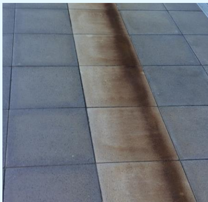
Figure 2: Concrete staining due to incorrect management of runoff from weathering steel wall directly above
